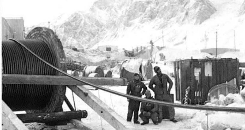
Ziehen eines der 4 Tragseile, Ø 62 mm, Gewicht je 40 Tonnen, Bruchlast pro Seil 425 Tonnen. Pulling one of the four 27/16" track cables. Each track cable weighs 40 m. tons and has a breaking strength of 425 m. tons.
